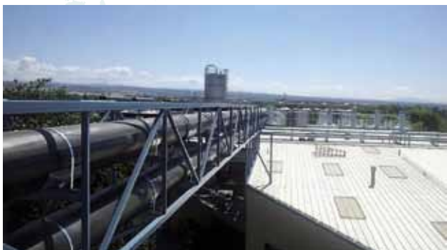
Cool Fit ABS Plus installed outdoors for the cooling unit of all the fermenting cellars at the Sierra Nevada Brewery.
